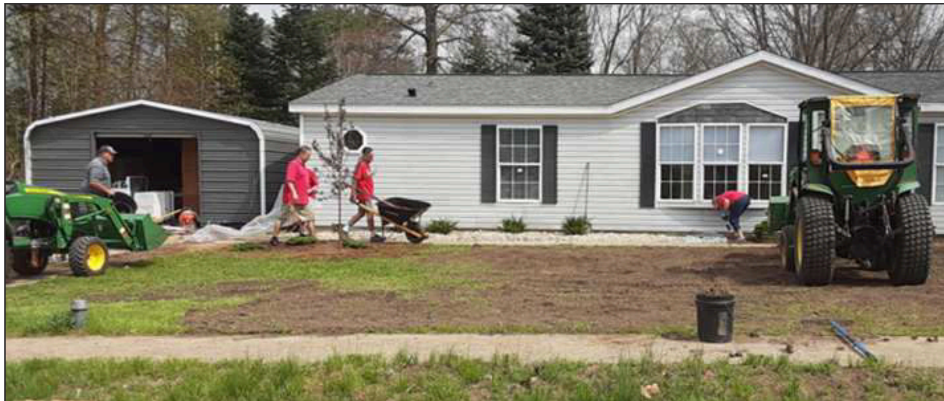
A crew from Keller-Williams Realty in Holland put the finishing touches on the landscaping at one of the houses Hank renovated for People Helping People in Pullman.
